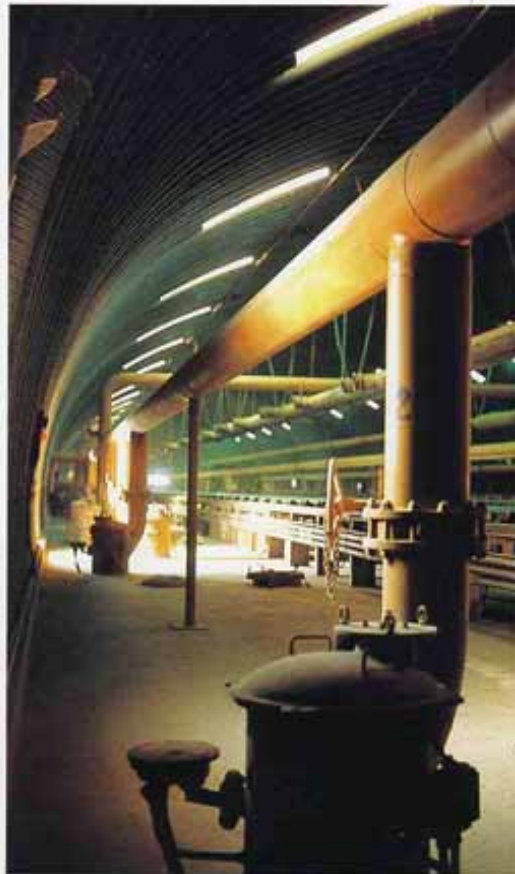
훈증소독설비 / Fumigation Facility
