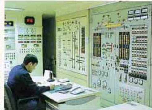
중앙통제실 / Central Control Room
